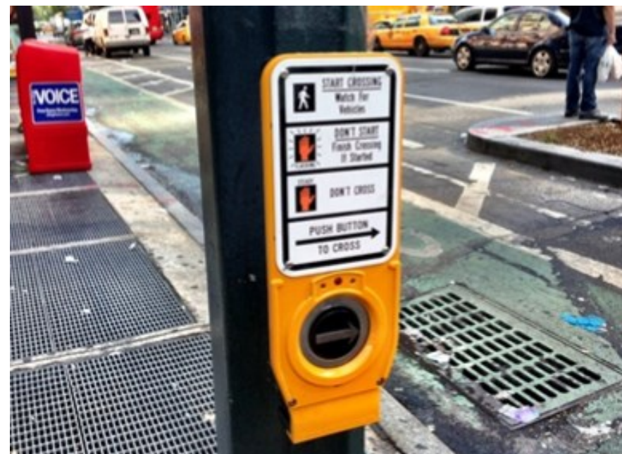
Accessible Pedestrian Signal Push Button
