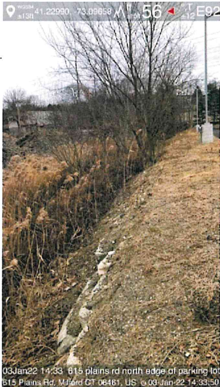
Photo 4 facing east fill over boulder / block retaining wall with loose soil.
