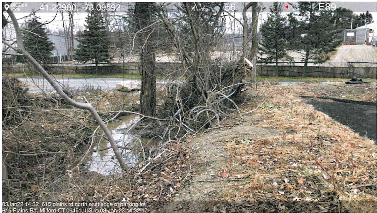
Photo 2 intermittent watercourse from site facing east. Unprotected loose soil along slope.
