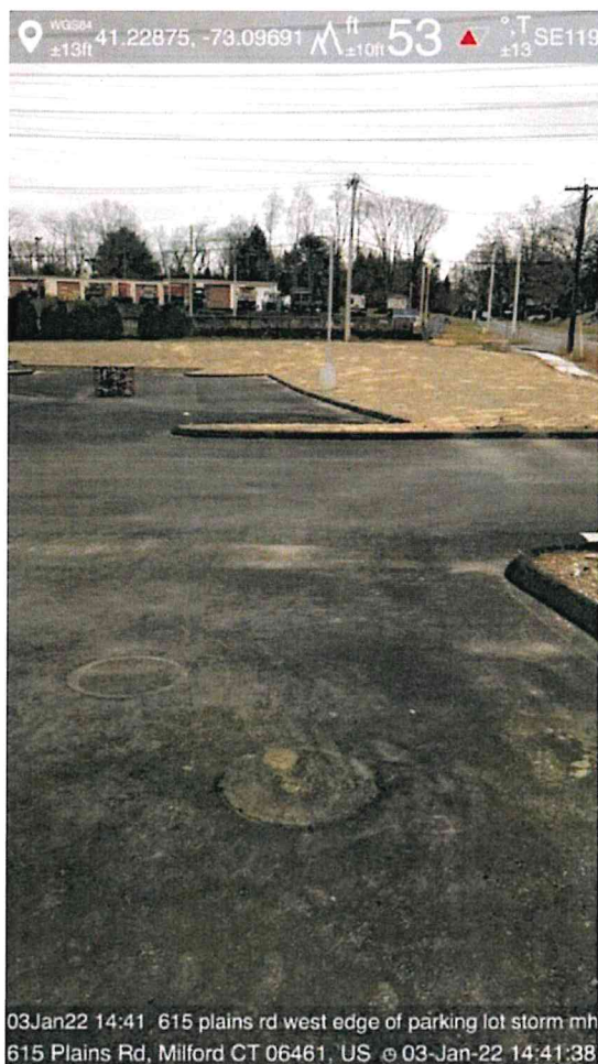
Photo 7 Facing southeast towards Raton Dr. Two(2) manholes for stormwater system.
