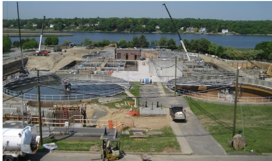
Beaver Brook WWTP Image: carlincontracting.com
