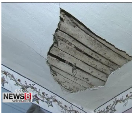
Minor damage in Plainfield, CT, after a small quake in January
